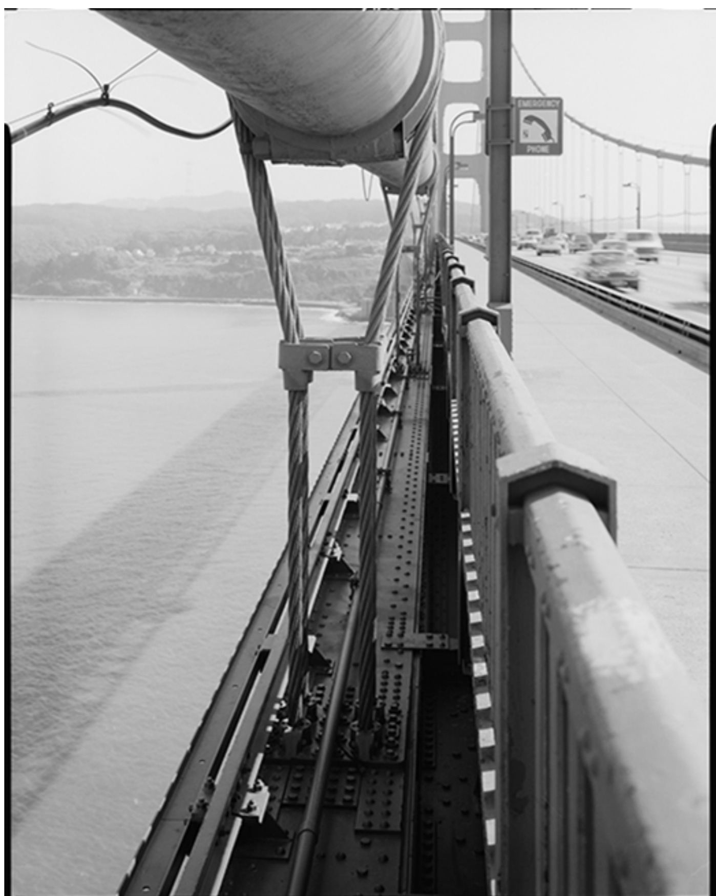
Detail View Showing Connection of Suspender to Floorbeam. Jet Lowe, photographer, 1984. Golden Gate Bridge, San Francisco, California. Historic American Buildings Survey/Historic American Engineering Record/Historic American Landscapes Survey. Prints & Photographs Division
